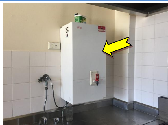
Photo 12. Ground level, kitchen, hot water boiler – suspected SMF internal insulation
