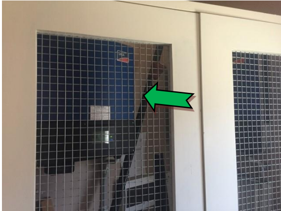
Photo 7. Ground level, main hall, behind stage, electrical backing boards – suspected non asbestos-containing bituminous backing boards
