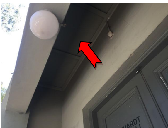
Photo 5. Exterior, southern elevation, fire exit, awning – assumed asbestos-containing fibre cement sheeting
