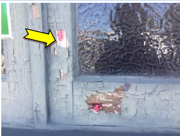
Photo 23. Exterior, throughout, window frames – lead-containing white lower paint systems
