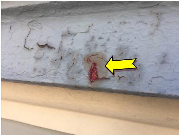
Photo 21. Exterior, throughout, walls – lead-containing lower white paint systems
