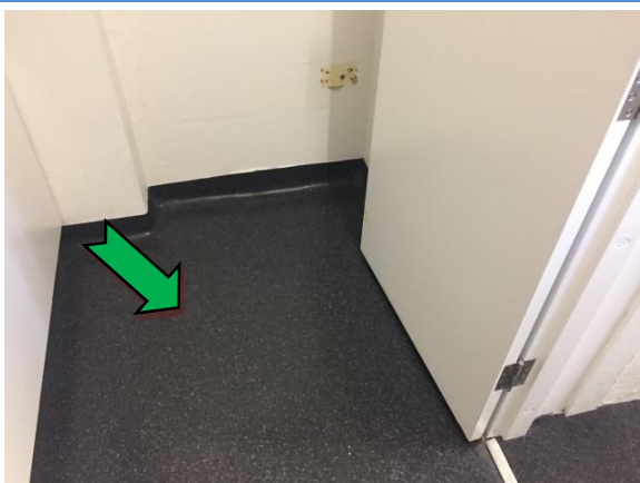
Photo 11. Ground level, Inner West Council offices, kitchen, lunch room & security room, floor covering – suspected non asbestos-containing black vinyl sheeting
