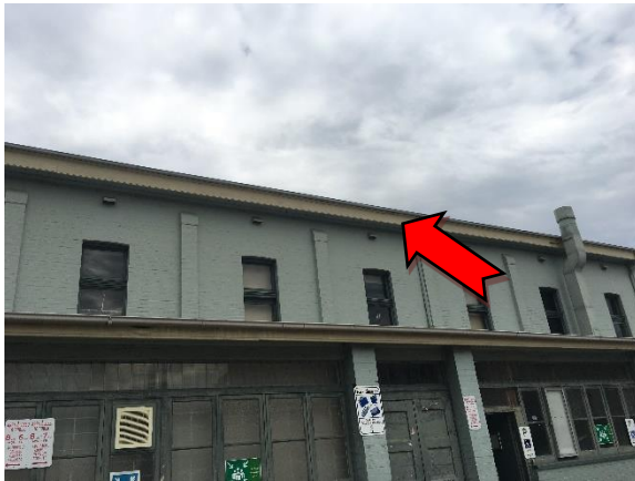
Photo 3. Exterior, main hall, surrounding eaves – suspected asbestos-containing fibre cement sheeting
