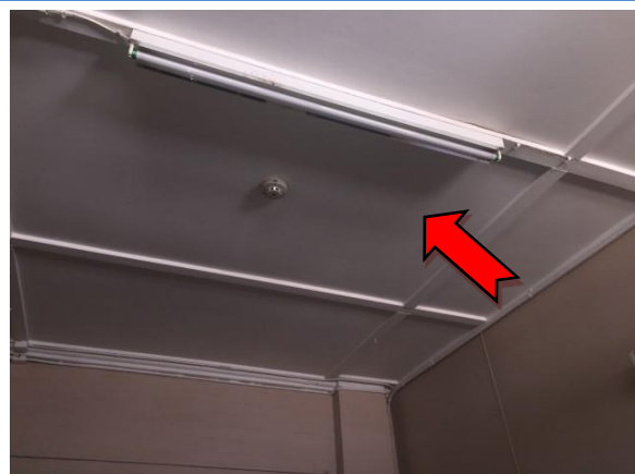
Photo 6. Ground level, eastern extension (excluding kitchen), ceiling lining – asbestos-containing fibre cement sheeting
