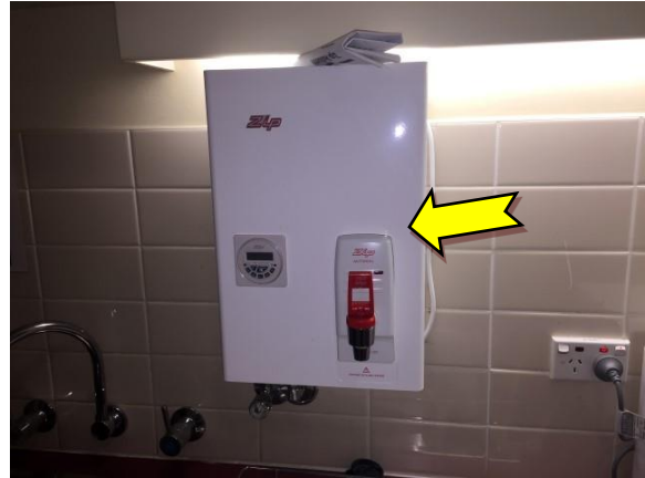
Photo 14. Ground level, north-east kitchen, south wall, hot water boiler – suspected SMF internal insulation
