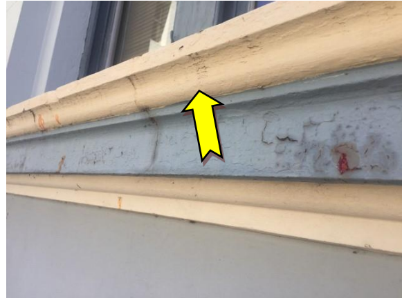
Photo 20. Exterior, throughout, walls – lead-containing light yellow upper paint systems
