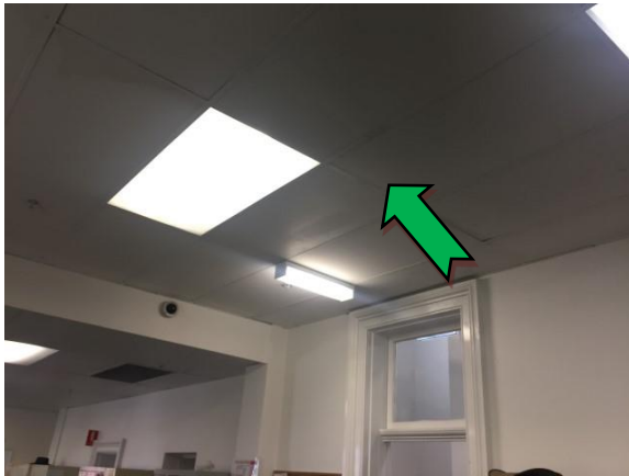
Photo 15. Ground level, Inner West Council Offices, north-west office, ceiling lining – suspected non SMF compressed ceiling tiles
