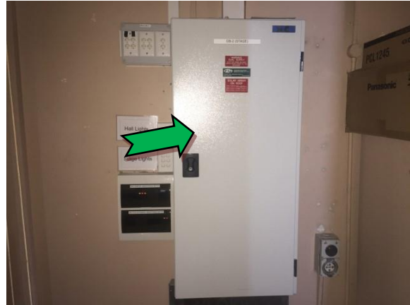
Photo 8. Ground level, main hall, switchboard – suspected non asbestos-containing bituminous backing boards
