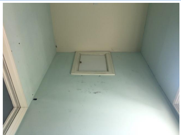
Photo 24. No access – ceiling space to level 1 female bathroom (access hatch at on wall)
