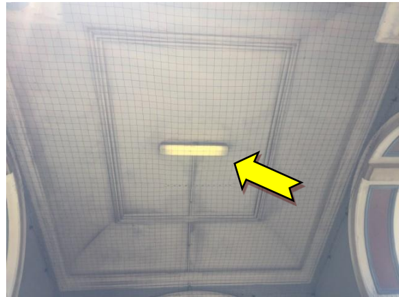
Photo 16. Exterior, western elevation, entrance – suspected PCB-containing single tube fluorescent light fitting
