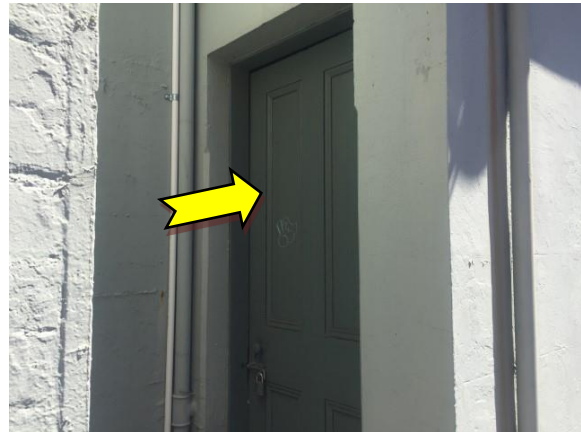
Photo 22. Exterior, throughout, walls – lead-containing dark green paint systems
