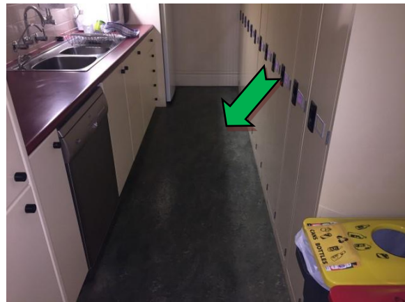
Photo 10. Ground level, councillors lounge, floor coverings – suspected non asbestos-containing green vinyl sheeting
